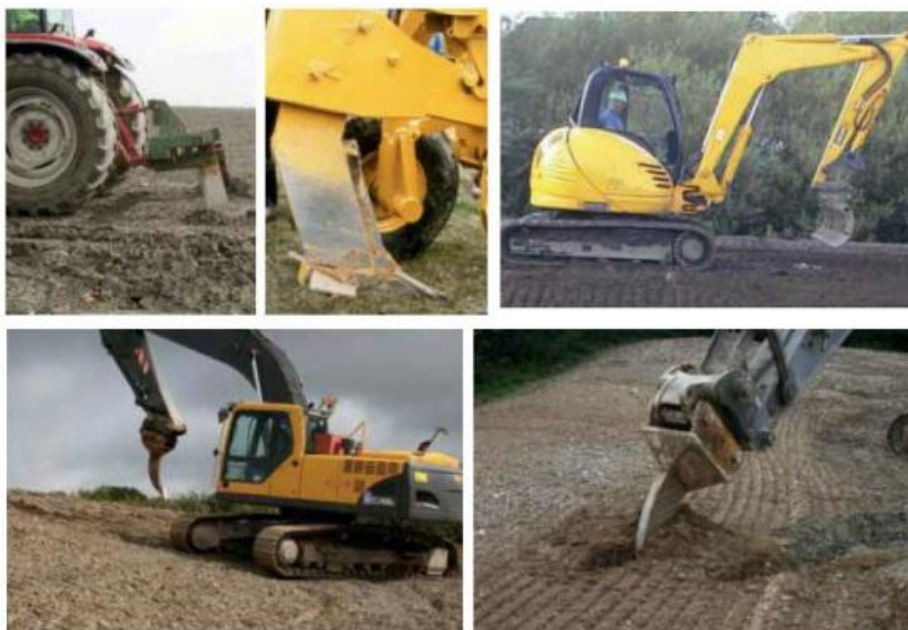
Figure 3-4: Top: (left to right) Tractor-drawn tines; Large winged ripping tine; Topsoil rake on 3-tonne excavator. Bottom: Single ripper tooth relieving compaction to a depth of 600mm
